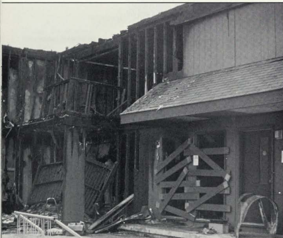
The boarded doorways are those of apartments destroyed in the 1981 fire.
