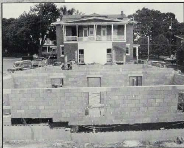
A large addition is being added to the rear of the Alumni House.
