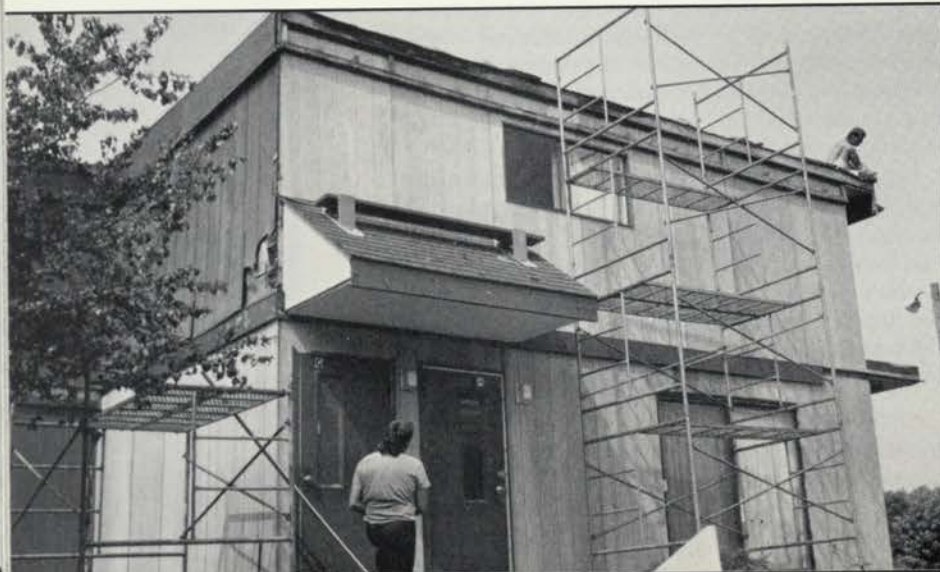
The dingy dark red siding is being replaced by natural colored wood.
